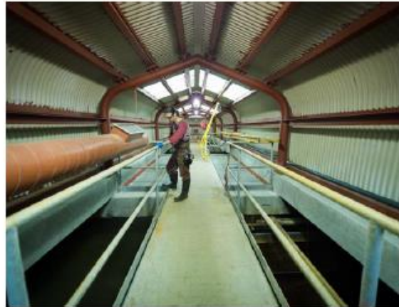
Primary clarification. Photo: Mike Crane
