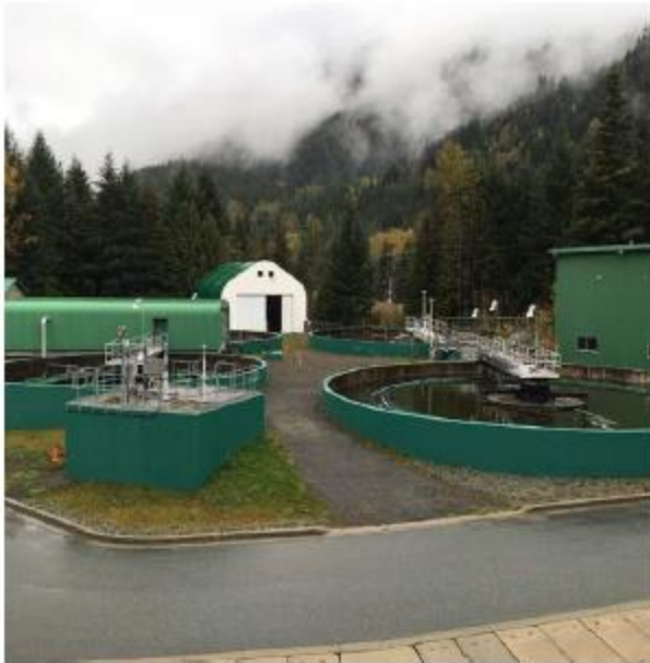
Secondary clarification overview. Photo: Trish Browning
