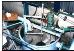
Flocculation Mixing Tank
