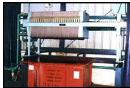
Hydraulic Sludge Press
