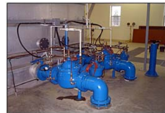
Backwash Control Valves
