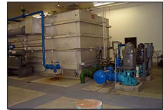
Filtered Water Pumps
