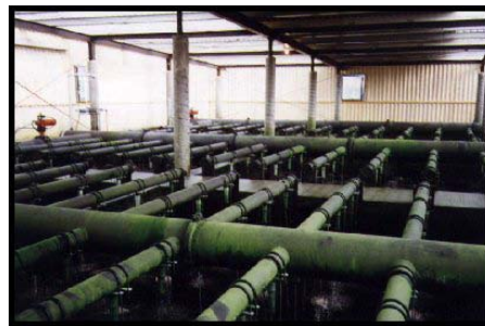
Distribution Pipes Above Biofilters
