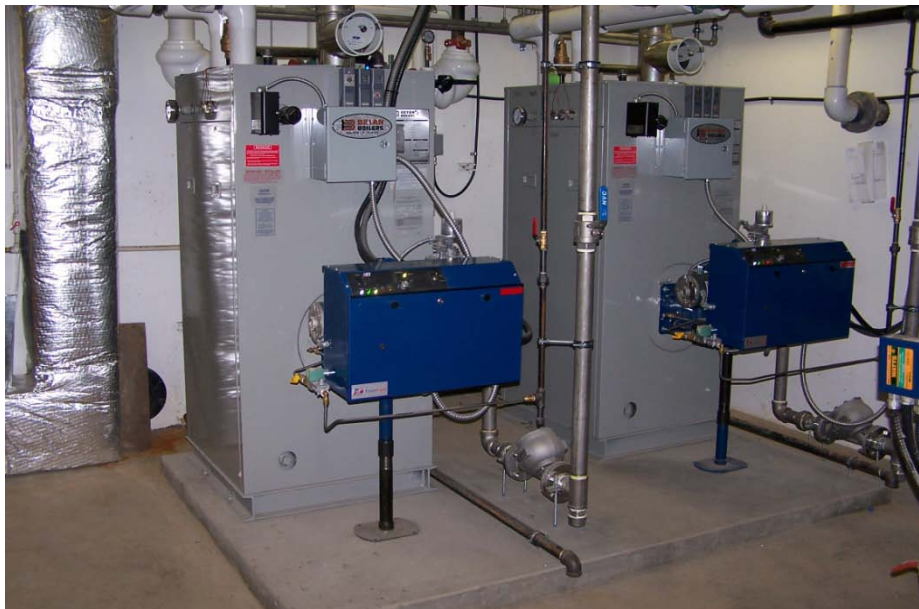
Photo of new methane boilers
